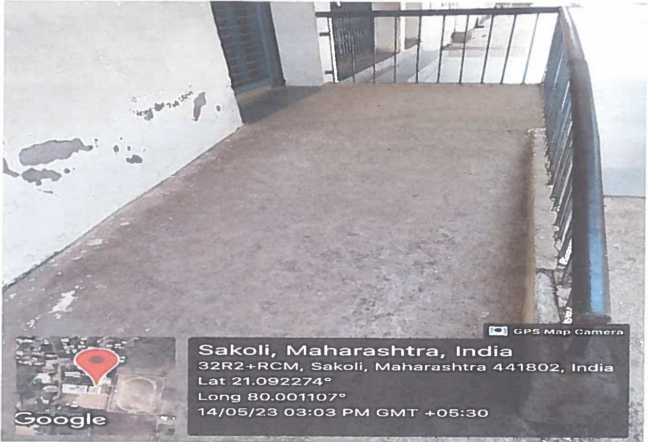
Ramp for Disabled person
